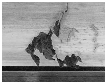
Point Surface Origin (PSO) spalling.
